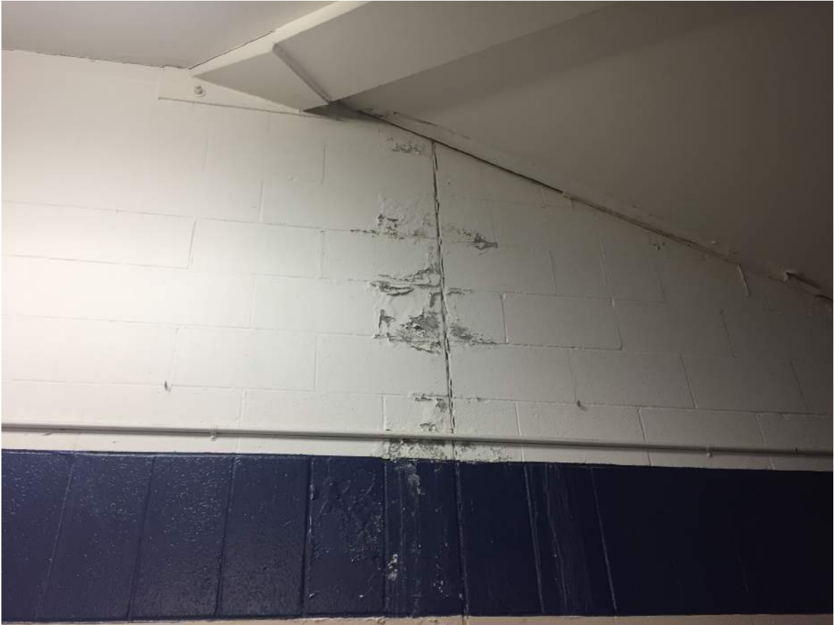
Photo 1: Moisture intrusion at the intersection of the lobby roof and CMU wall.
