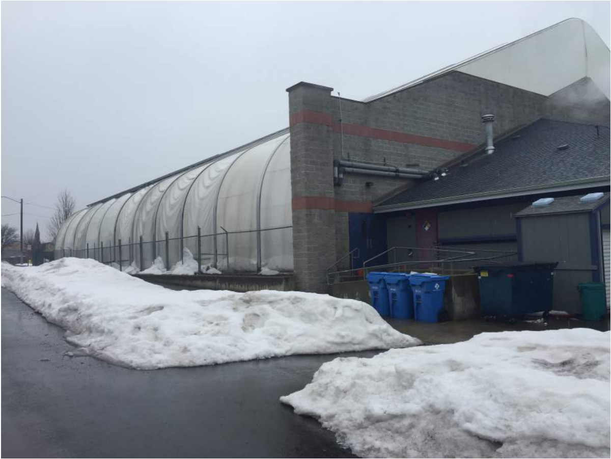
Photo 4: Stretched and sagging pool cover.
