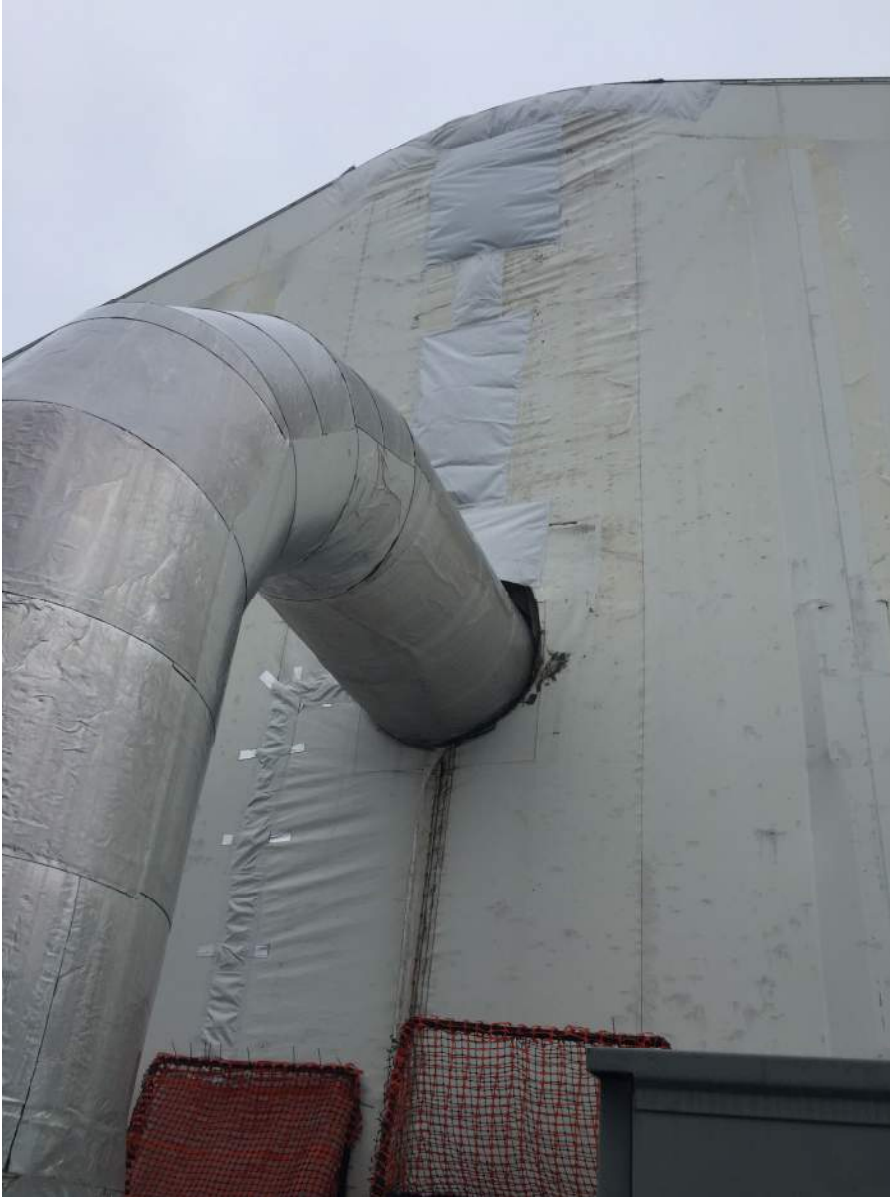
Photo 3: Damaged and repaired pool cover.
