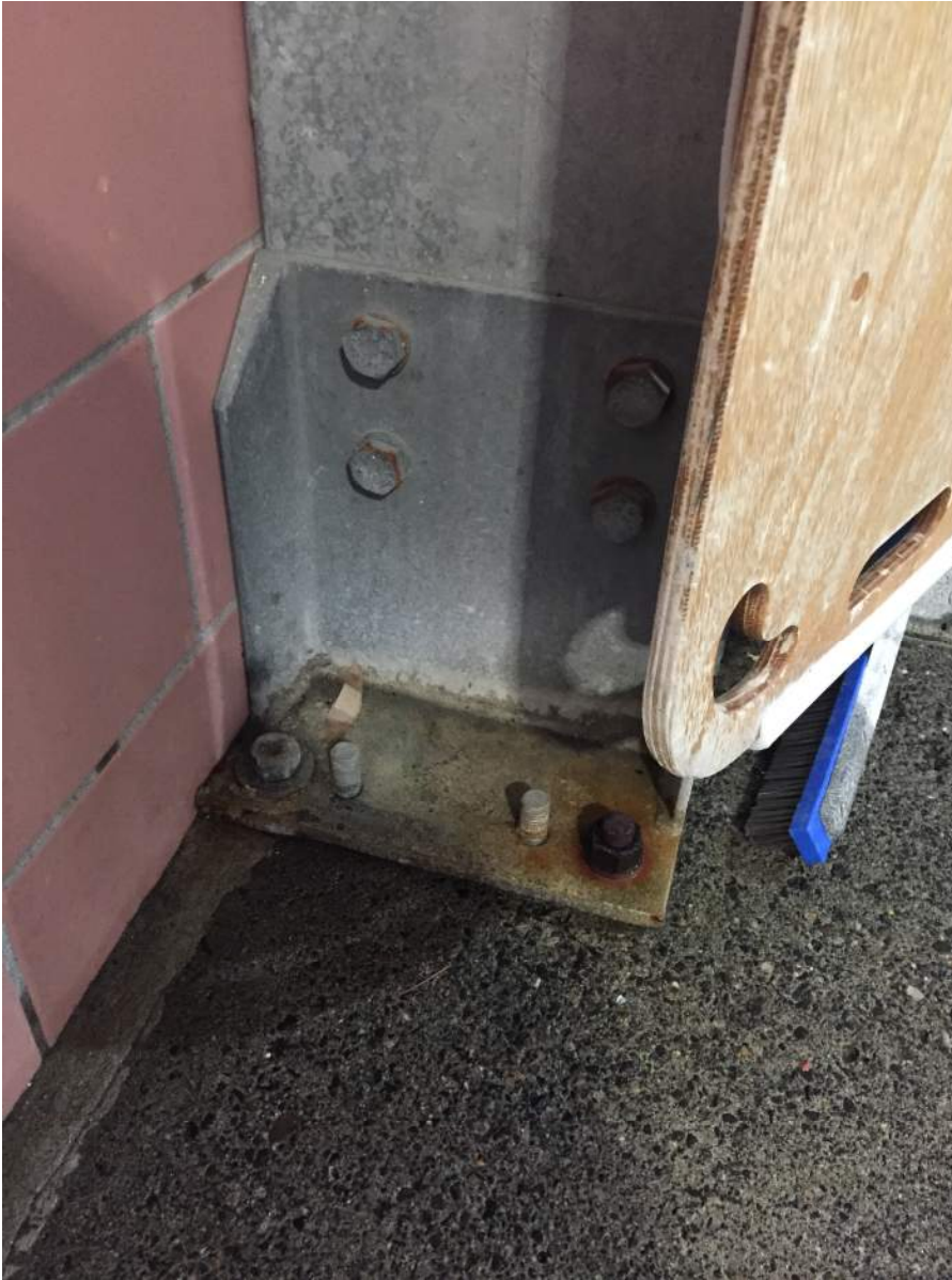
Photo 2: Corrosion and missing fasteners.
