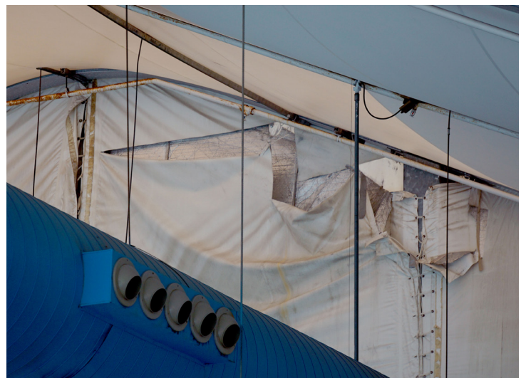
The tent wall on the west end is being held together by rope and zip ties.
