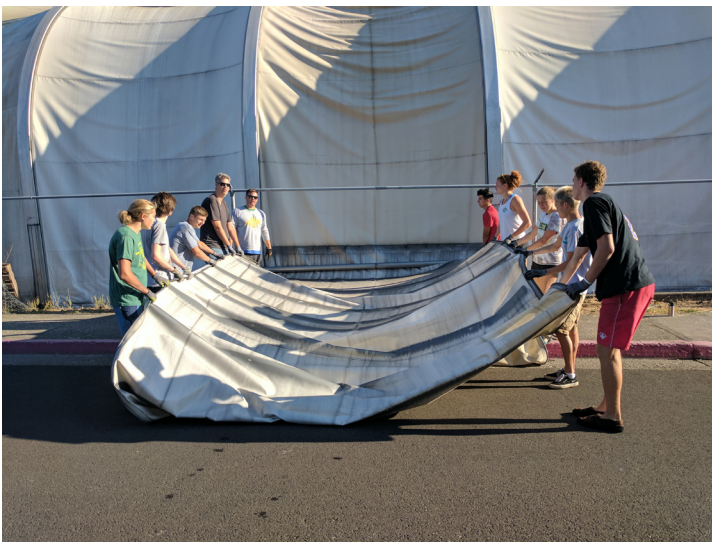
Panel replacements have become a common occurrence at the Hood River Aquatic Center.
