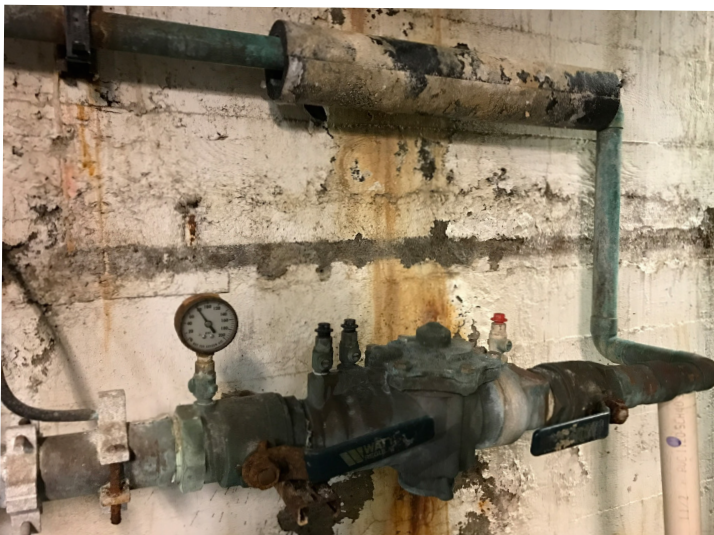
This deteriorating piping is a strong indicator of the condition of the thousands of feet of plumbing underground.
